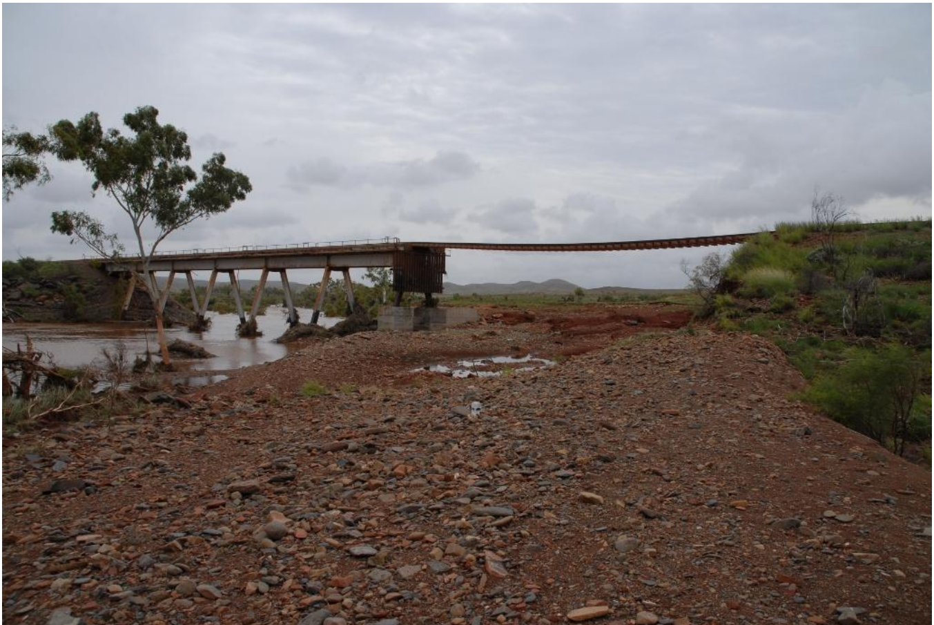
Washout on Hamersley Iron Dampier Tom Price main line at 76km Western Creek Bridge showing extent of damage having the embankment washed away leaving track suspended in mid air February 17th. Photo Justin Parry
