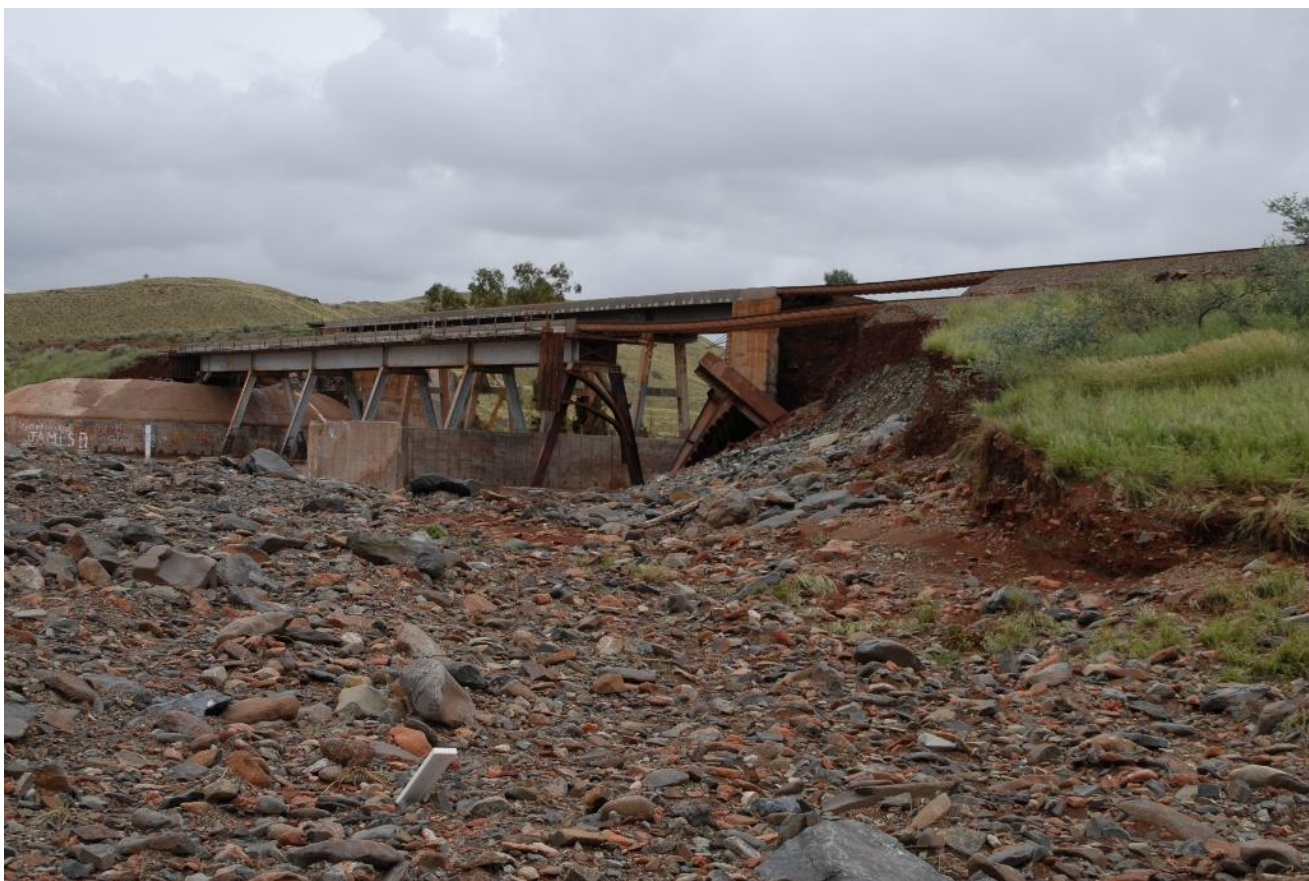
Another washaway occurred at 85km on Dampier Tom Price line at Harding River Bridge where the embankment of both bridges was washed away again suspending tracks in mid air February 17th. Photo Justin Parry
