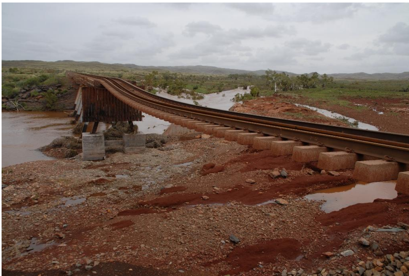
Track is suspended in mid air on Western Creek Bridge February 17th showing where the water just washed the embankment away following torrential rain in the Pilbara. Photo Justin Parry
