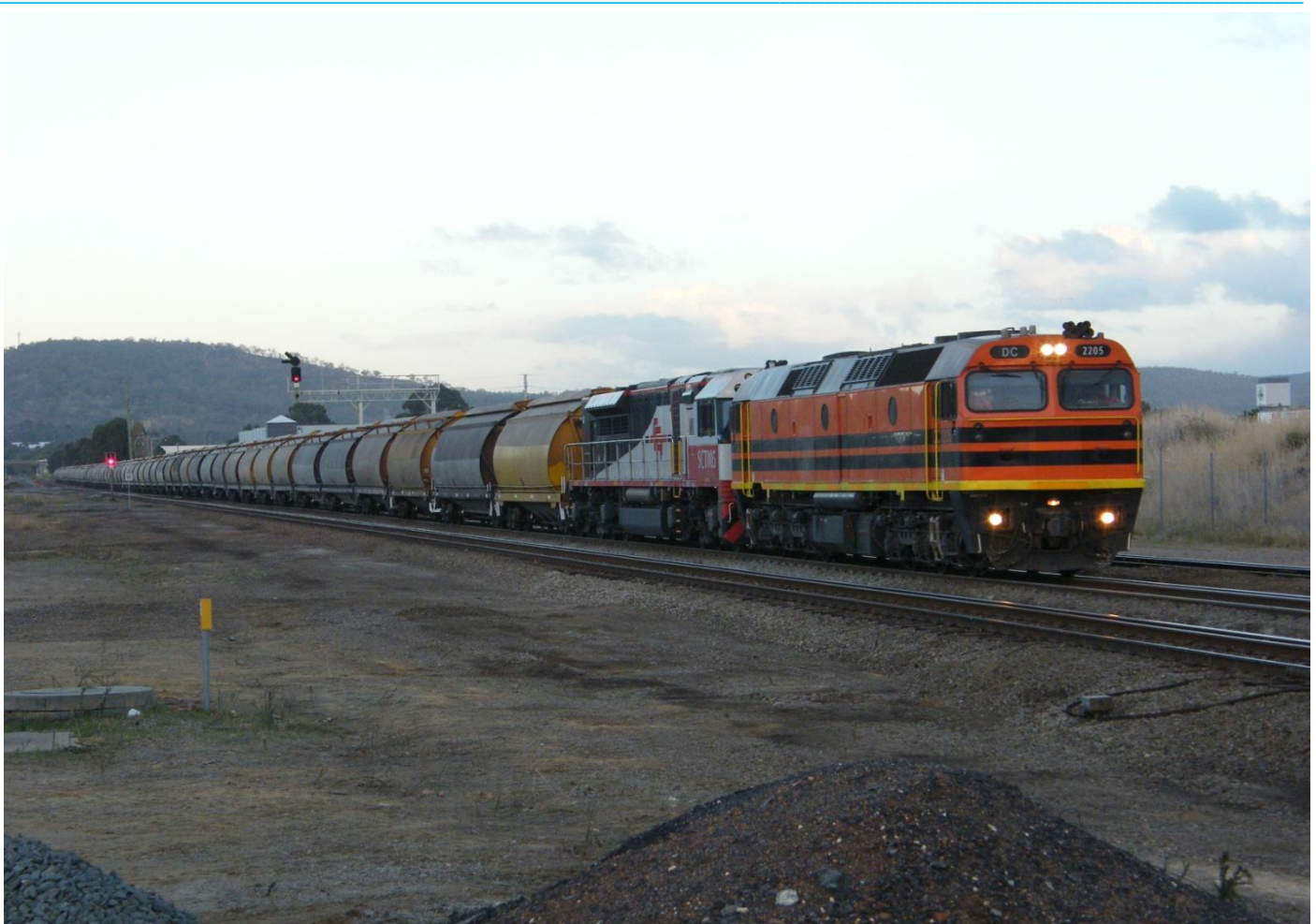
DC2205 Avon Yard shunter returning to Forrestfield & SCT005 run 4056 grain train in evening of June 10th over the newly laid concrete sleepers as part of track upgrading at Midland. Photo Jim Bisdee
