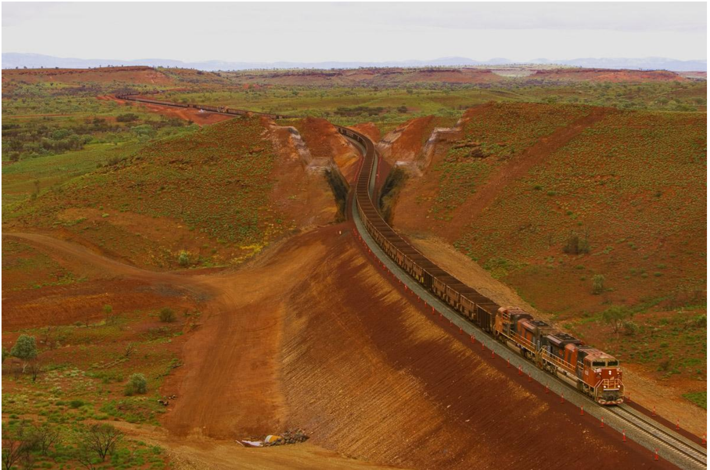
4350 and further SD70ACe on April 7th lead first loaded ore train of 330 cars two more SD70ACe and two AC6000 through cut 5 on new BHP Billiton Iron Ore Chichester Deviation. Photo John Stephens
