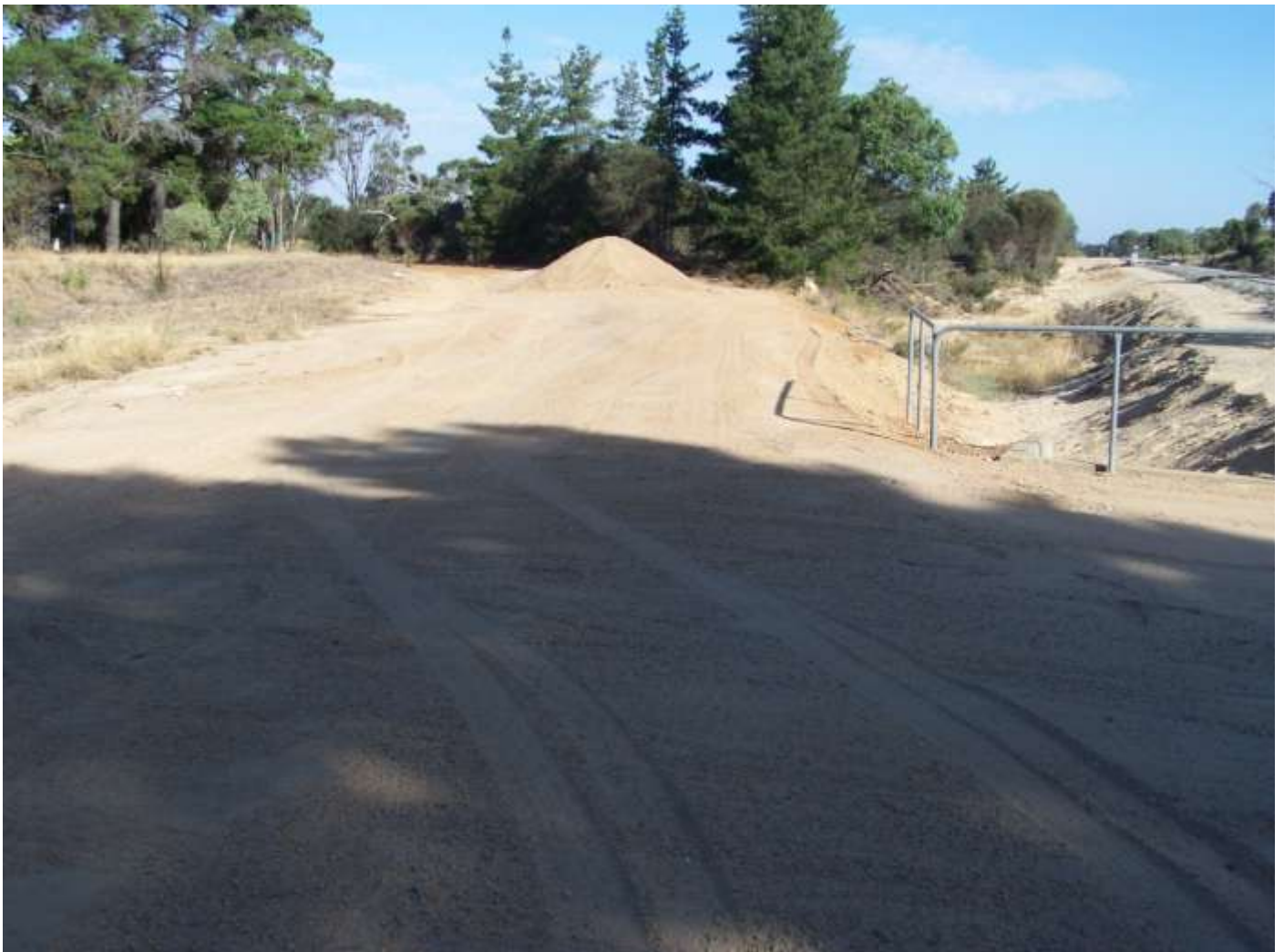
Gnowangerup line connection been removed line is in distance February 23rd. Both photos Daryle Phillips
